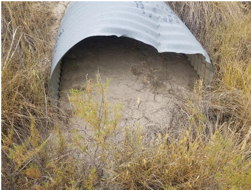
Photo 11. Culvert full of dried silty material exhibiting desiccation cracks.
